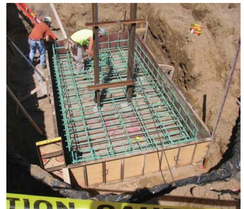
Downtown Steam Vault
