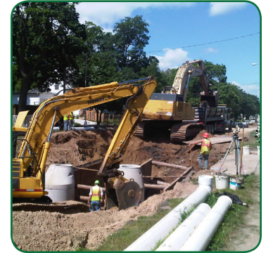
Sanitary and sewer installation
