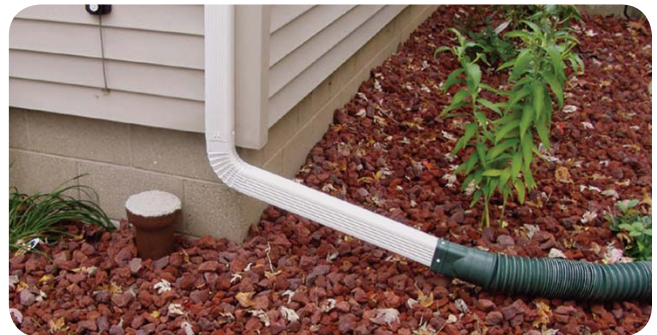
Redirected Downspout and Plugged Riser Pipe
