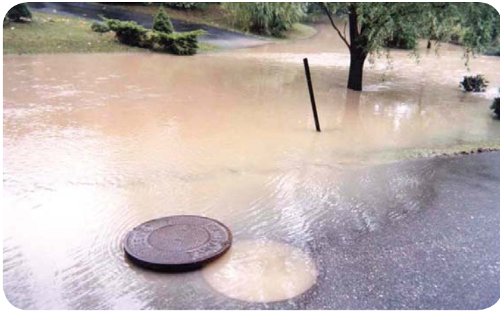
Surface Flooding and Sanitary Sewer Overflow
